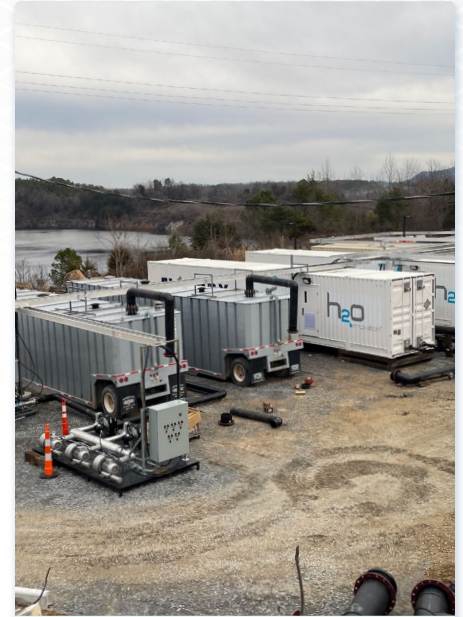
Water Treatment Plant: Water is being pumped from the water treatment plant at a rate of 2,500 gallons/minute and discharged safely into the Kings Creek.
